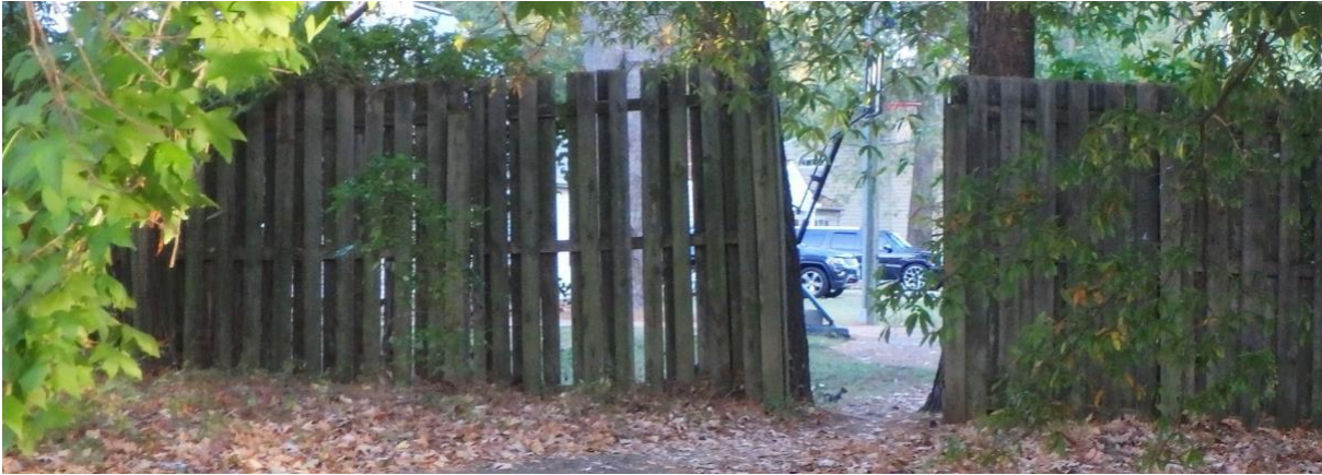
The opening in the fence next to the Coastal Community Church on Victory Blvd.
